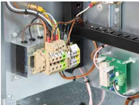
Fig 11 - incoming power terminals
